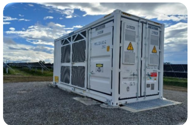
Transformer Station at Lauriston Solar Farm
