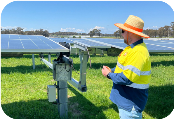
FRV worker standing next to solar panels that track the sun
